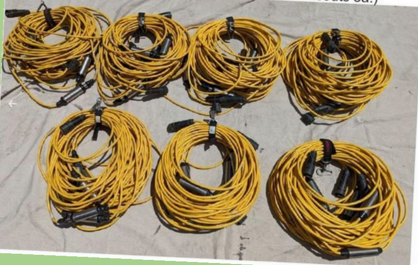
14 spread cables w/ 4 take-outs ea., 20-ft spacings (56 takeouts total, shown as 7 coils of 8 takeouts ea.)
